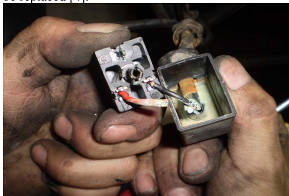
Fig. 10. Damage of cable [4]
