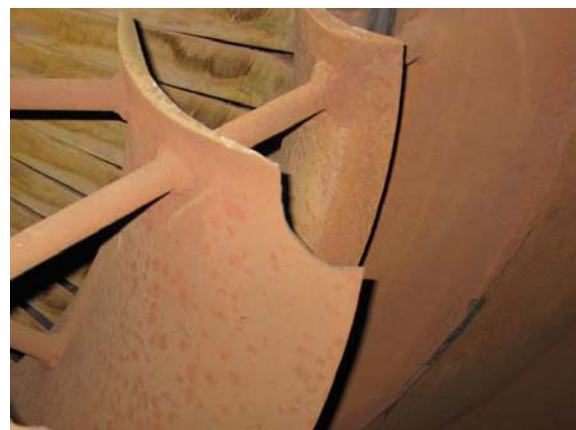
Fig. 5. Photographs of damaged guide fences; in the upper photo, arrows indicate loose welded joints (1) and the guide fence that has fallen off (2); lower photo shows damaged guide fence edge
