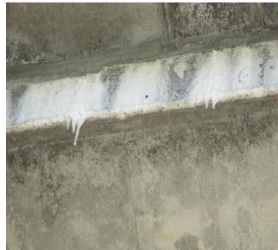
Fig. 6. Concrete leaching of over-bridge constructions
