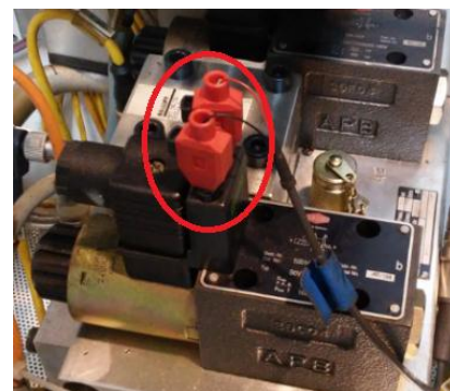
Fig. 1.5. Connection to the coil of PSV
