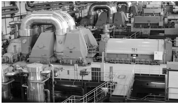
Fig. 4. Photo of the 230 MW turbine-generator unit (source: Wikipedia)
