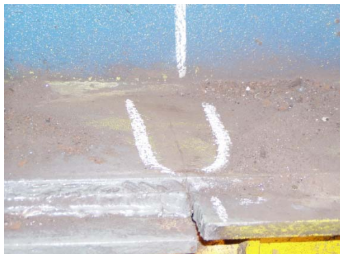
Fig. 9. The same fatigue crack, view from above
