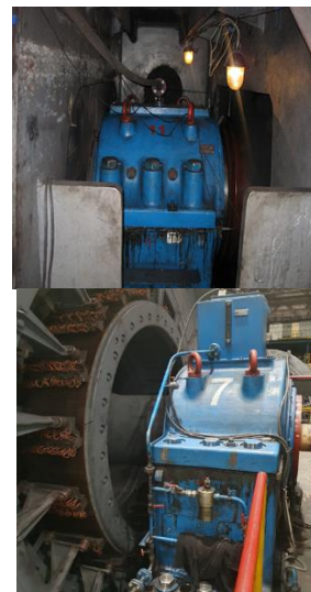
Fig. 1. Rolling mill drive motor plain bearings
