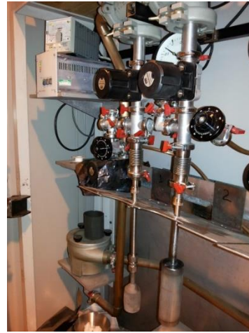
Fig. 5. The degassing equipment
