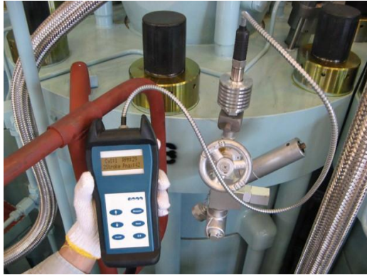
Fig. 3. EPM-XP application on MAN B&W two-stroke diesel engine built under license by Kawasaki Heavy Industries [7]
